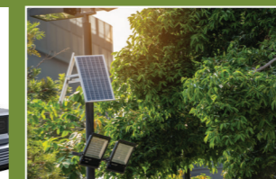
Solar street lights
